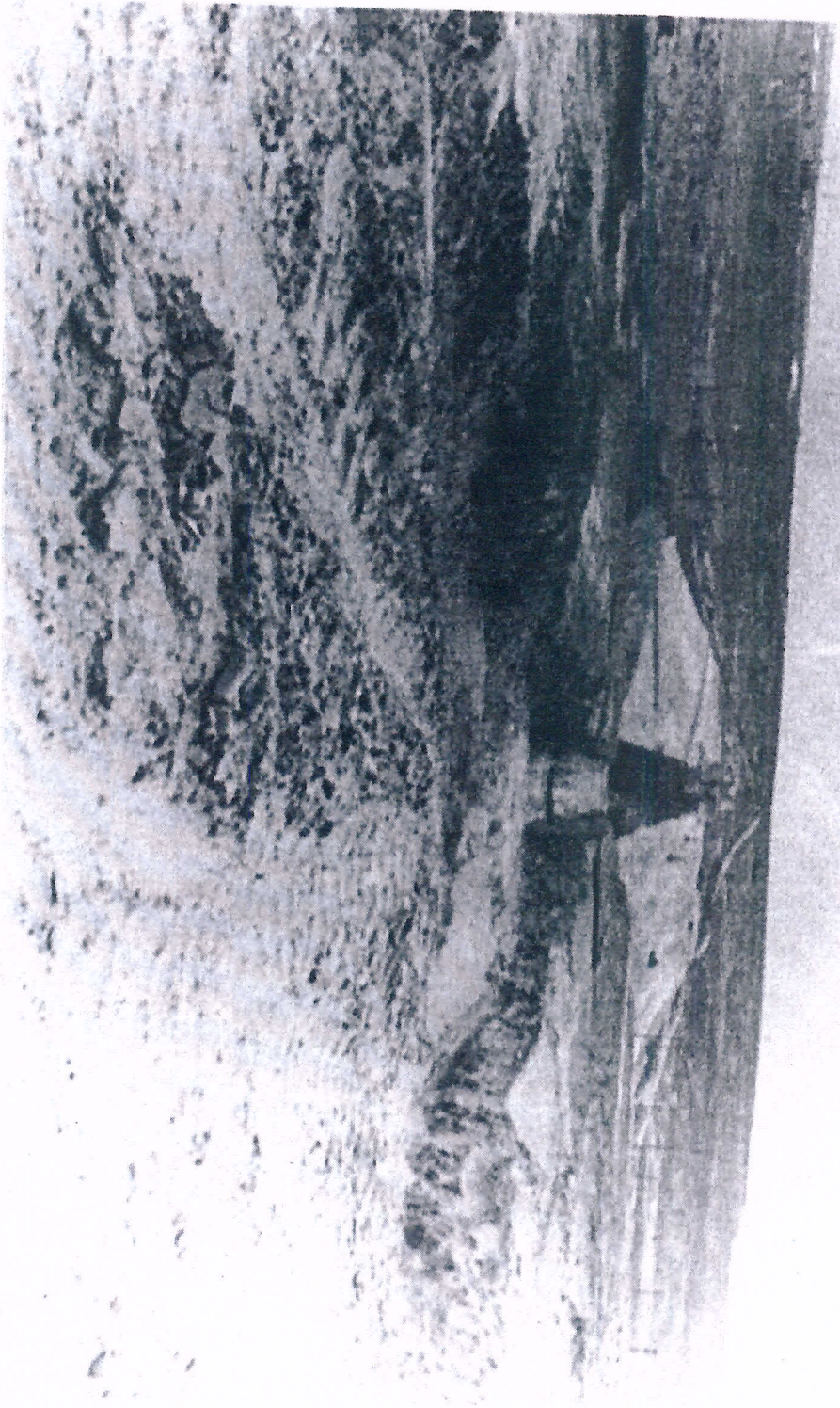
Excavation for Morgan Lake Dam. To the right of the cut (East) will become Morgan Lake. 5/17/61
